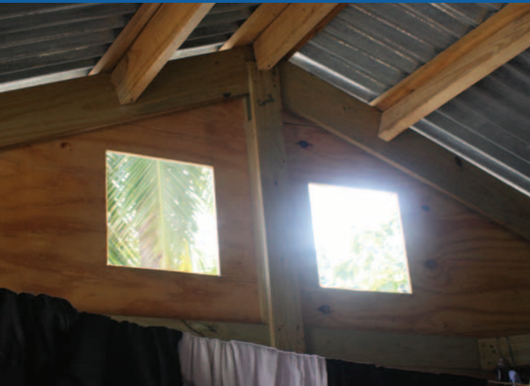
The original ventilation holes beneath the roof let in too much rain. Staff observed that community members often covered up these holes. Photo by Niek de Goeij/CRS.
