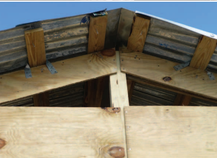
CRS Haiti changed the square holes to triangular holes so that beneficiaries would not need to choose between fresh air and dry shelters. Photo by Niek de Goeij/CRS.
